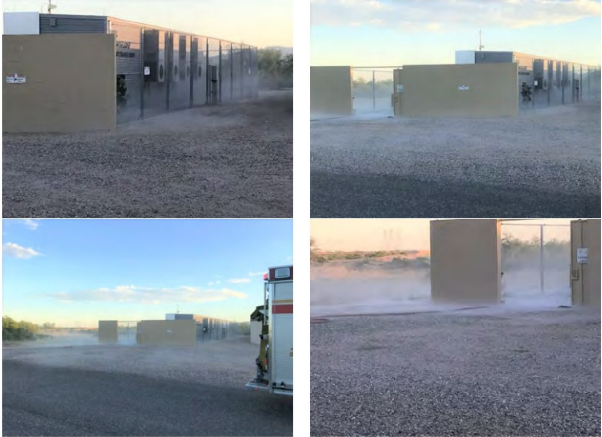
Figure 10 Photograph taken during the Surprise, AZ battery energy storage system incident, showing a white fog along the ground. Photograph from Surprise Fire-Medical Department. 83
