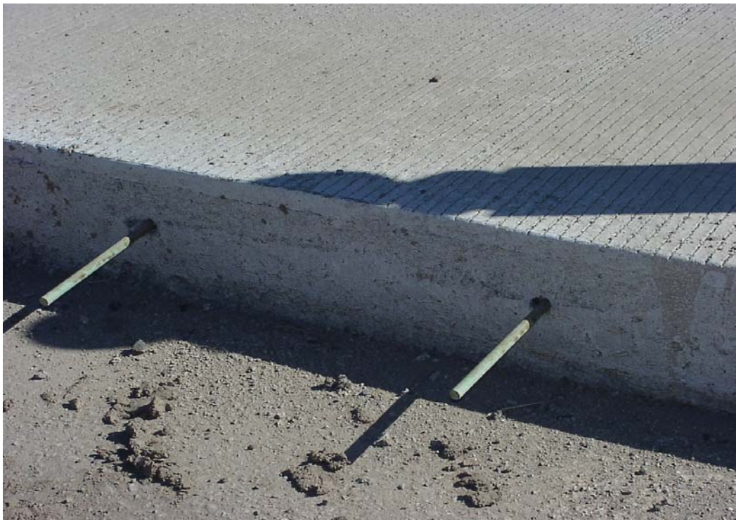
Figure 3.18. The dowel bars for the connection of the new slab with the existing slab
