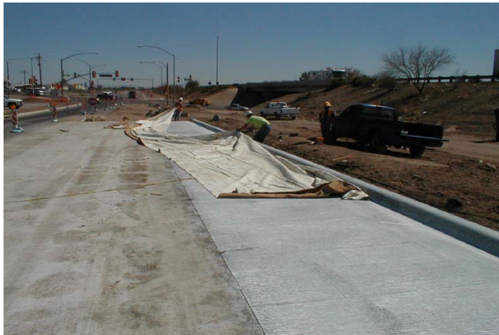
Figure 3.22. Covering of the freshly poured slab to reduce the moisture loss during seven days moist curing process
